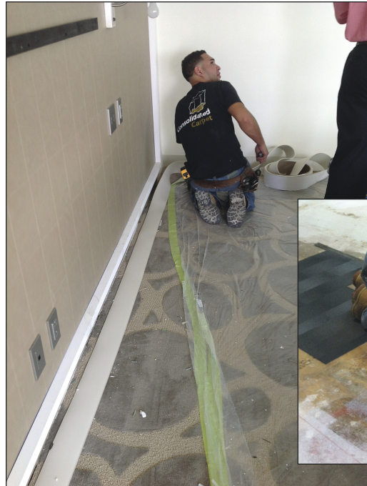
Left: Installer Anthony Milazzo of Consolidated works with cove base at New York's Millennium Hotel, while Jimmy Kickel, below, installs modular carpet at Maybank in New York.
